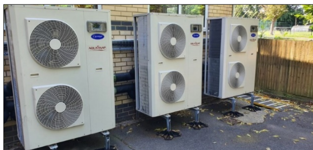
Caption: Air source heat pumps installed at Moss Hall Nursery as part of PSDS3a.
